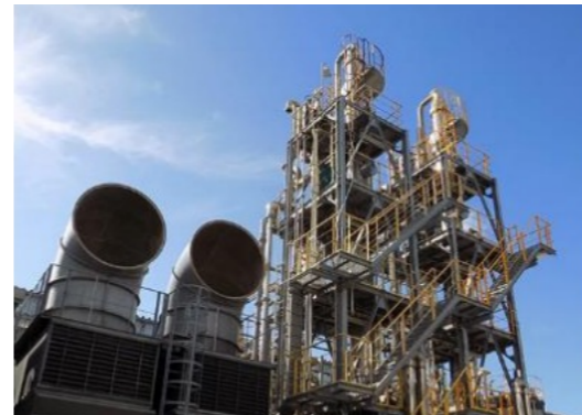
Ammonia stripping device at the Fukui site
